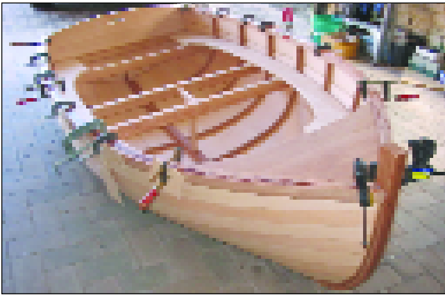
The aim is to construct the dinghy without seeing any screws on the inside. The final timber on the gunnel is glued and clamped covering all screws along this line.
